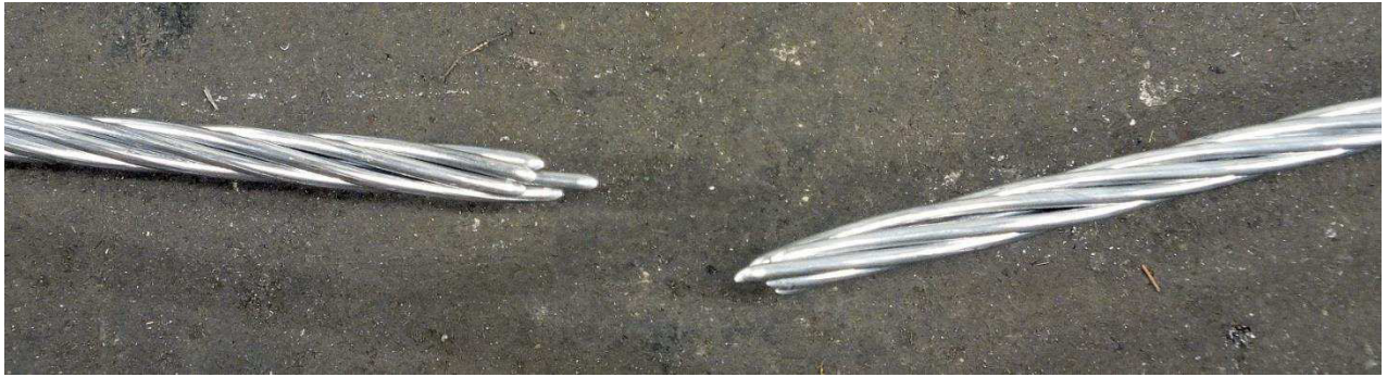
Fig. 2: Total breakage of the conductor in the free conductor span approximately 2,5 m from one end fitting.
